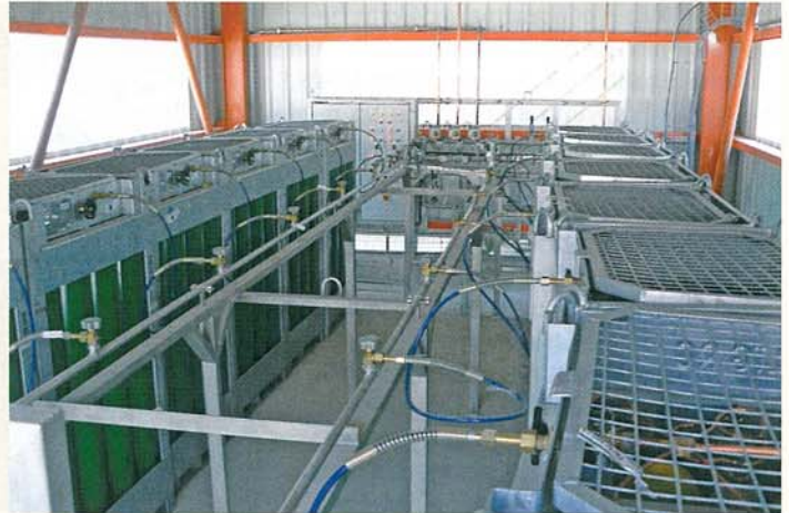
Fig. 3: Batteries of high pressure N 2 packs
